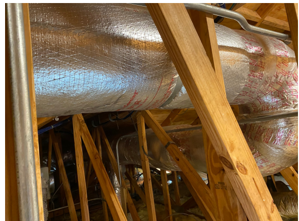
Site-wrapped supply ducts not inside the building thermal envelope must be insulated to R-8.
