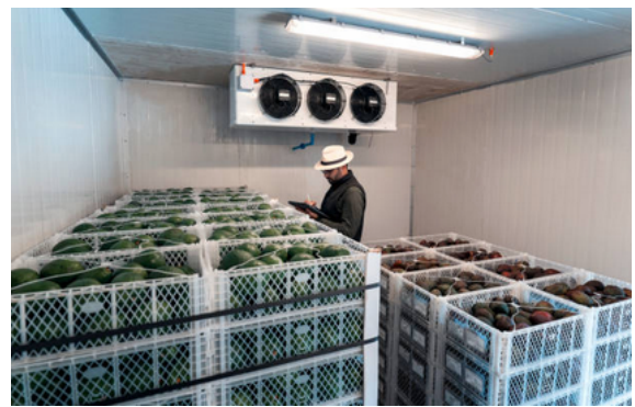
There are new lighting requirements for walk-in coolers and freezers.
